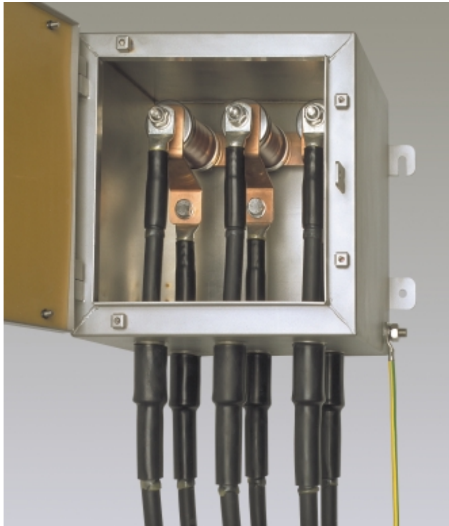
Link box installed with cross bonding cables
